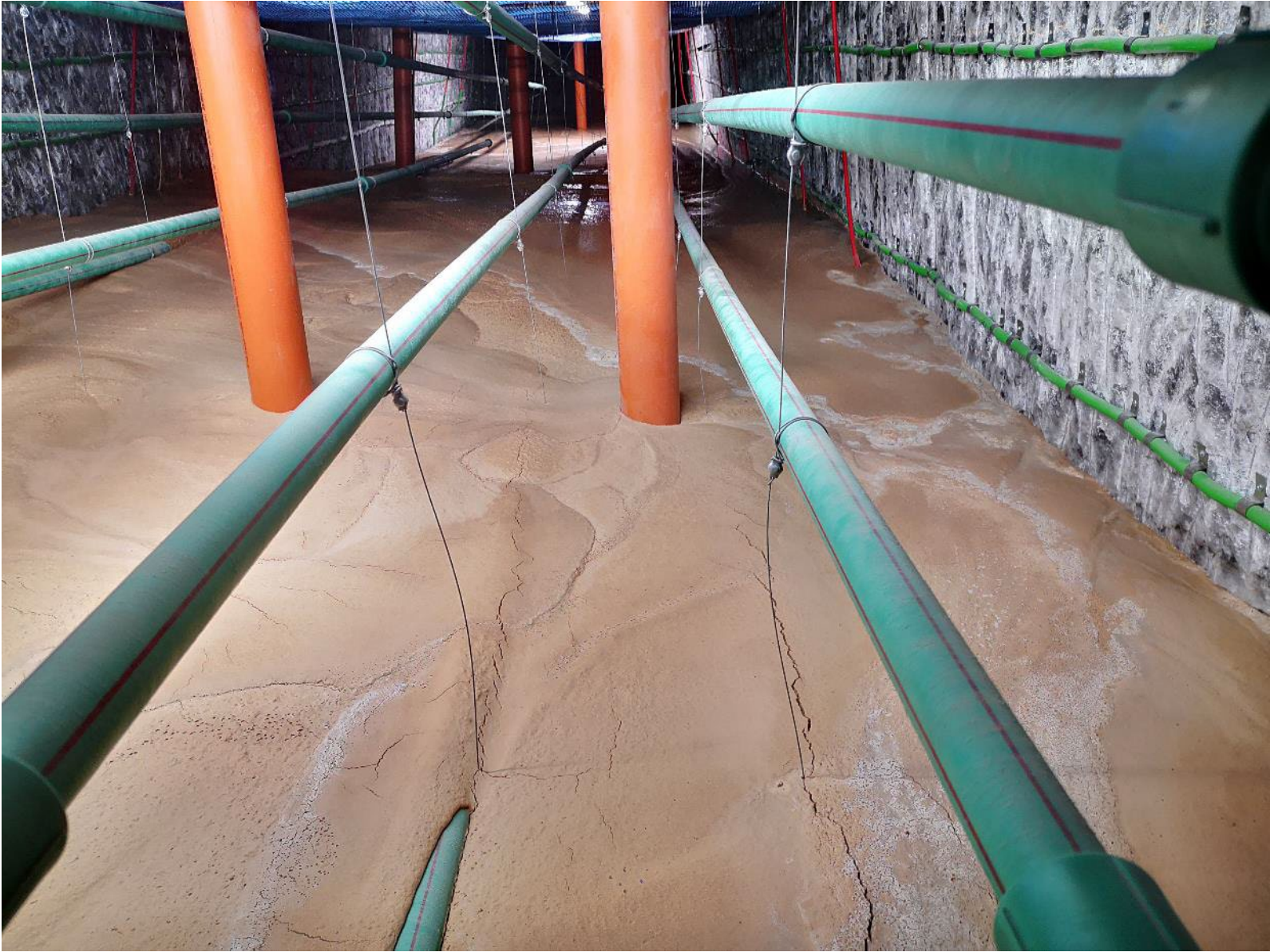
Crack formation after a 2 hours break; July 27 th 2021- 16:36
